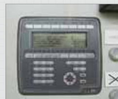
5 Control panel display
